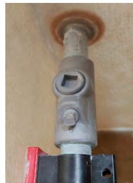
Shown installed from sump interior
