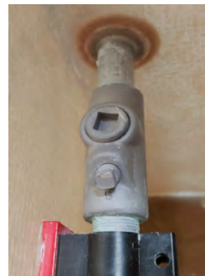
Shown installed from sump interior
