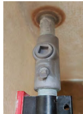
Shown installed from sump interior
