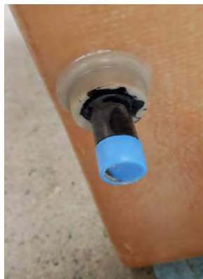
Shown installed from sump exterior
