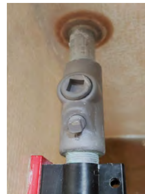
Shown installed from sump interior
