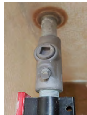
Shown installed from sump interior
